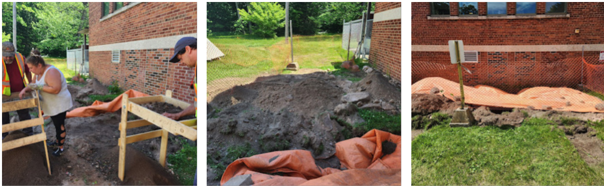
Figure 28, 29, 30 (left to right): Soil sifting after foundation exploration (in the 1B section of the site plan map).
